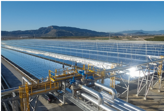
Source: Puerto Errado 2 liner Fresnel mirror power plant, Spain
